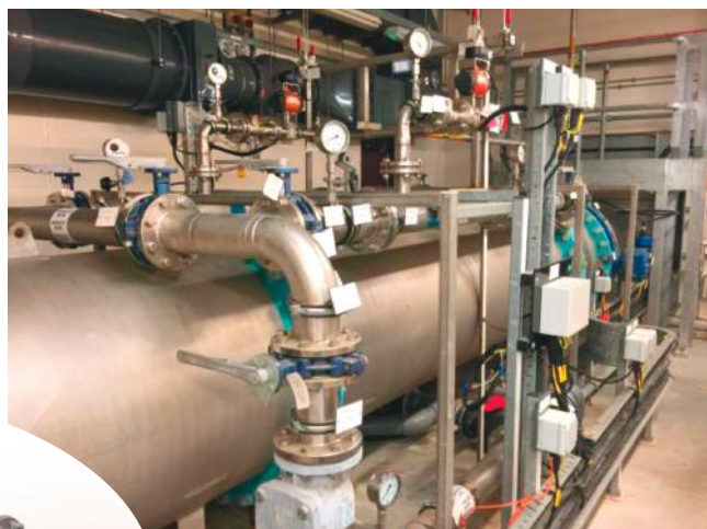
GDS installed at customer site
